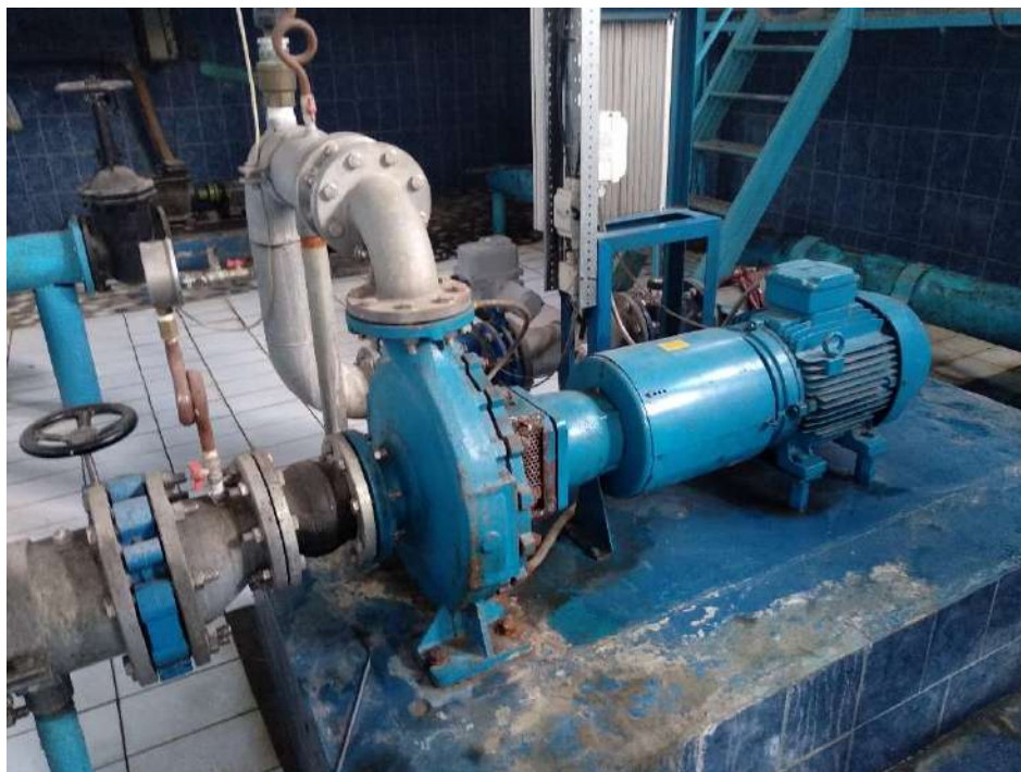
Figura 3-20: Pompa WEIR HL 125/100/400 (SP-05)
